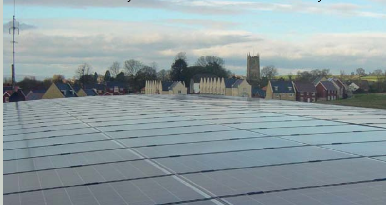
Our 50kW solar array on the roof of the Everhot Assembly Plant
